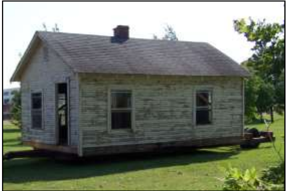
The exterior of the building will require paint, new windows, a porch and steps.
